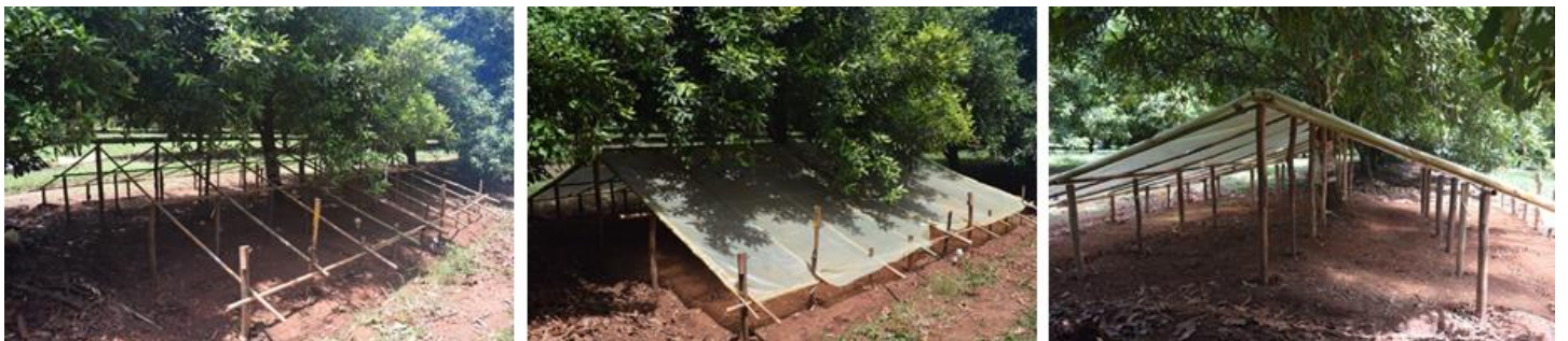
Above: Building of structures supporting throughfall-exclusion plastic covers under macadamia trees at Neuhof farm in Limpopo, March 2021. Photos: Thomas Bringhenti
